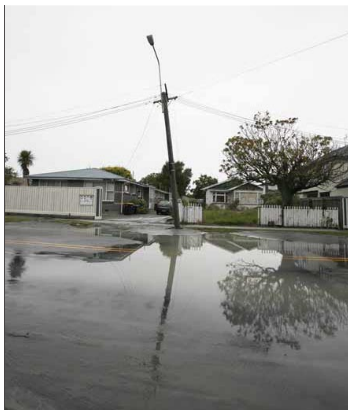
Flooding on Barbadoes Street, roads cracked, risen up, power poles on a lean. (Photo - NZPA / Pam Johnson)
