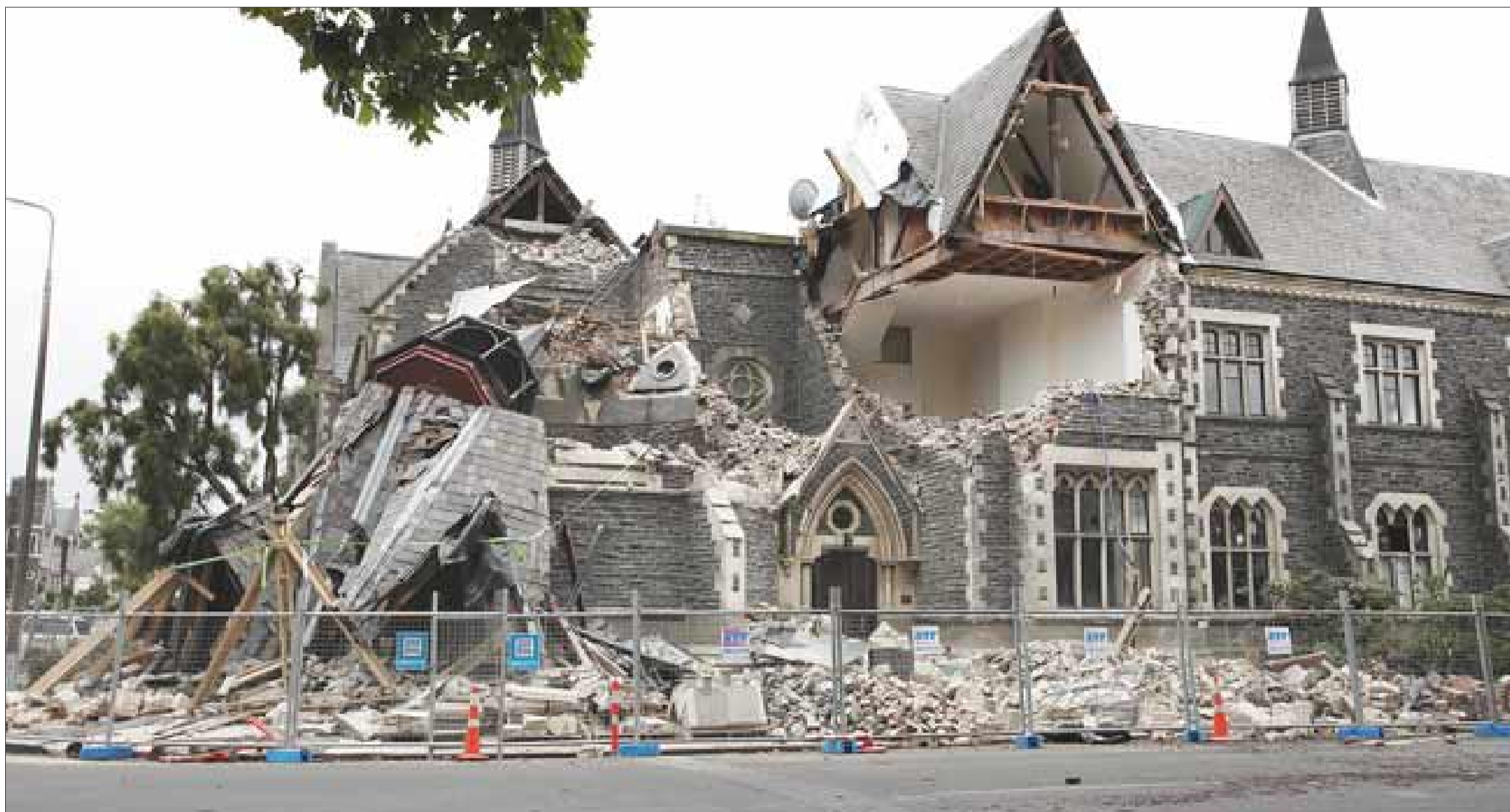
Cramner courts after earthquake. (Photo - NZPA / Pam Johnson)
