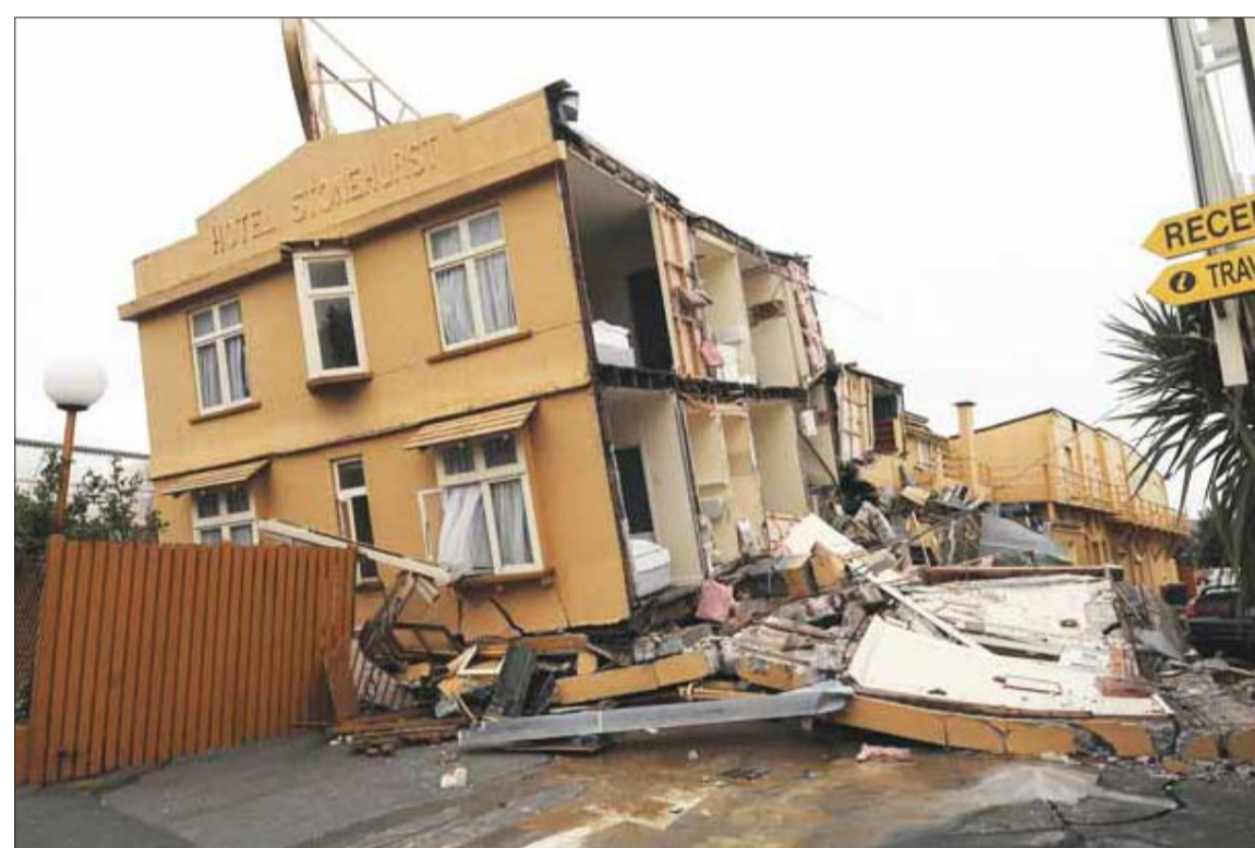
Hotel Stonehurst backpackers hotel lies wrecked in the inner city. (Photo - NZPA / David Wethey)
